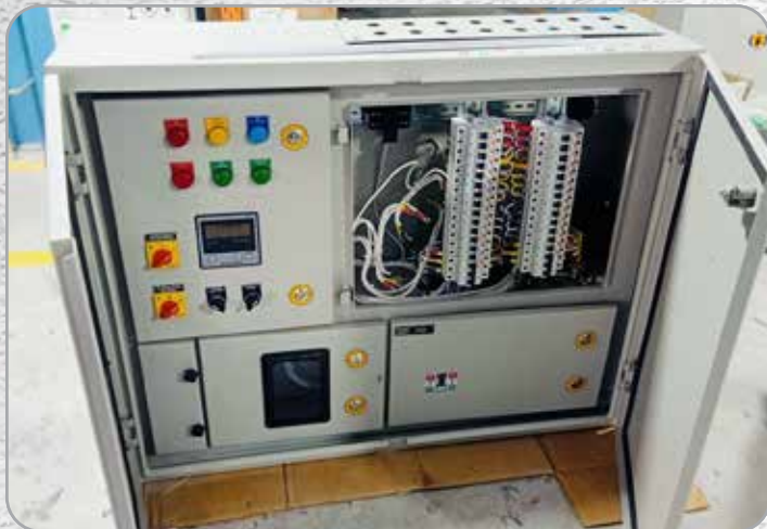
WHEN CURRENT GOES -THIS AUTO CHANGE OVER AUTOMATICALLY ON THE GENERATOR & WHEN THE CURRENT COMES IT AUTOMATICALLY OFF THE GENERATOR.
