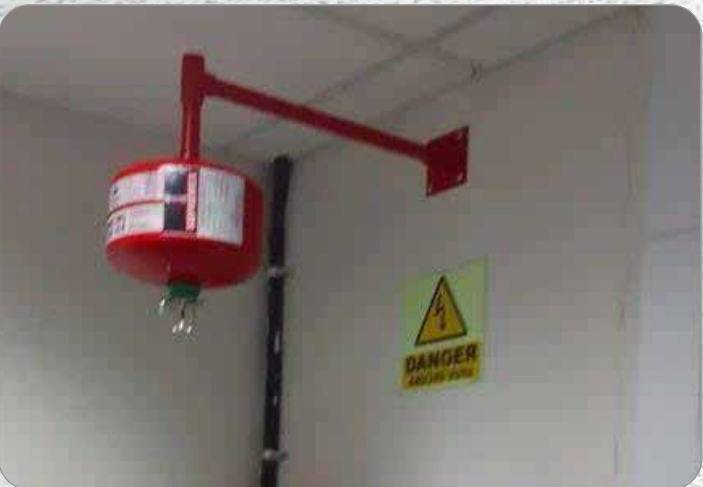
WILL BE FIXED IN EB PANEL BOARD AREA
