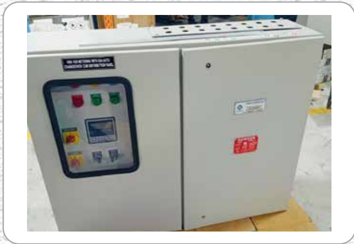
EACH VILLA WILL HAVE THIS 3 PHASE EB METERING WITH 63 AMS, AUTO CHANGE OVER CUM DISTRIBUTION PANEL BOARD
