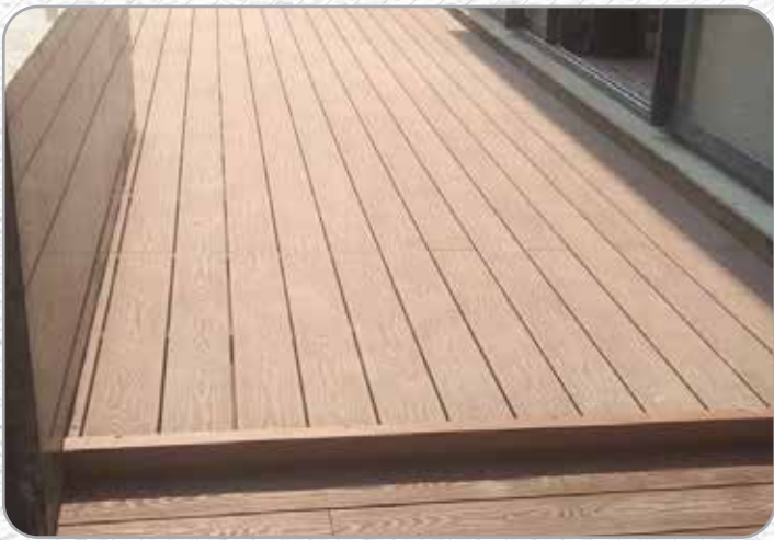
WPC USED IN WOODEN DECK AREA
