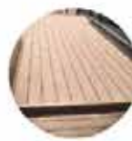
WPC - USED IN WOODEN DECK AREA.
