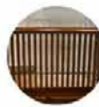
WPC - DECK HANDRAIL.
