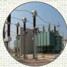
Common transformer yard
